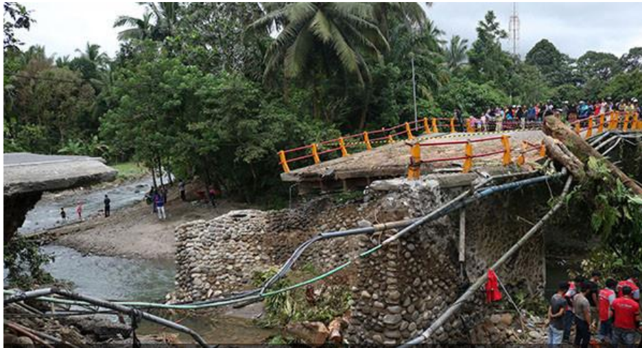
Figure 1. Damage to The Bridge that Connect Padang – Bukittinggi at KM 54 Kayu Tanam Source: Detik.news
