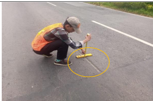
Figure 3. Damage to rut depth (observation result)
