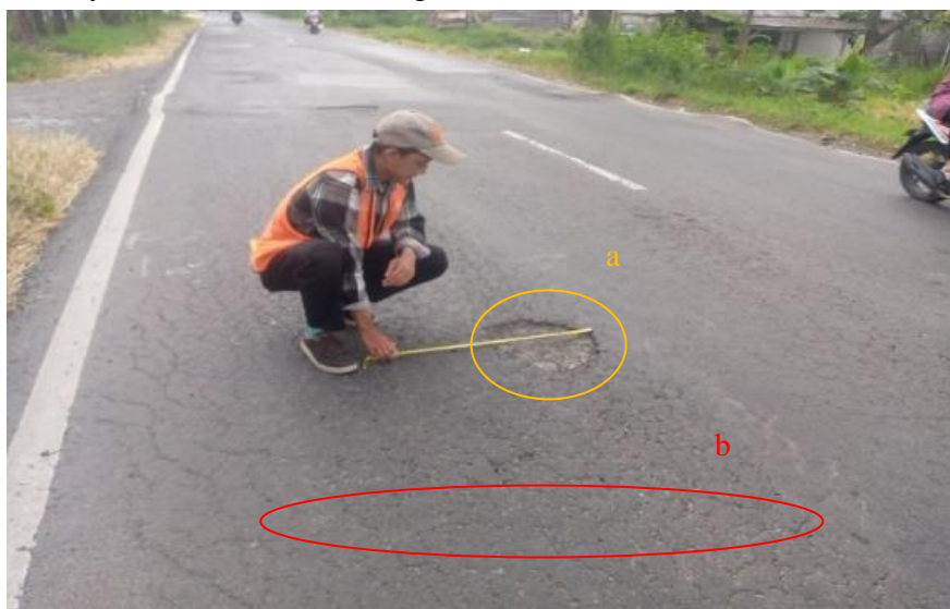
Figure 2. Damage (a) Potholes, (b) Crocodile Skin Cracks (observation result)
