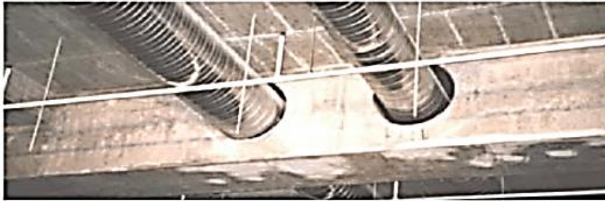
Figure 1: Example of a reinforced concrete beam perforated by a utility pipeline
